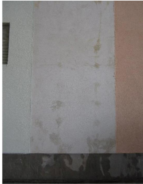
Figure 4: Detail of a Portion of the Specimen Showing Stains on the Surface of One of the Finishing Coats (Photo: ITC).
