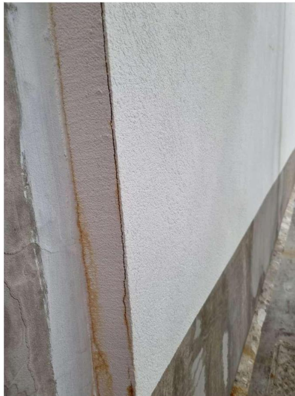
Figure 3: Detail of detachment between the render layer and the insulation along the edge of the specimen (Photo: ITC).
