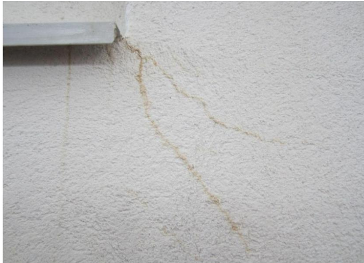
Figure 2: Detail of Cracks on the Surface of the Specimen Originating from the Corner of the Opening (Photo: ITC).
