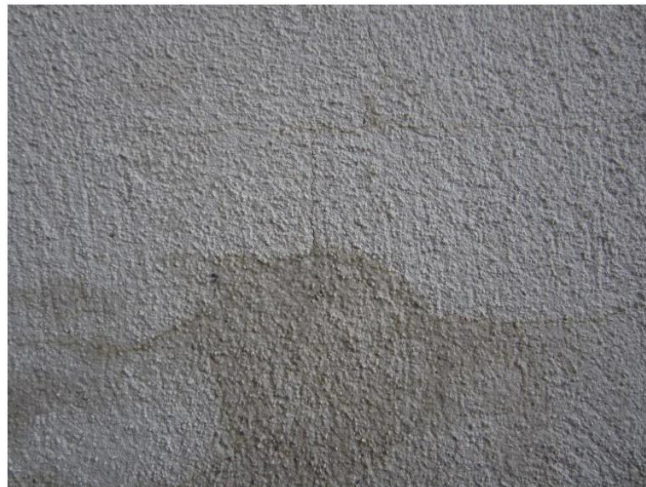
Figure 5: Detail of Surface Protrusion of the Fixing Anchor Head and Related Cracking (Photo: ITC).
