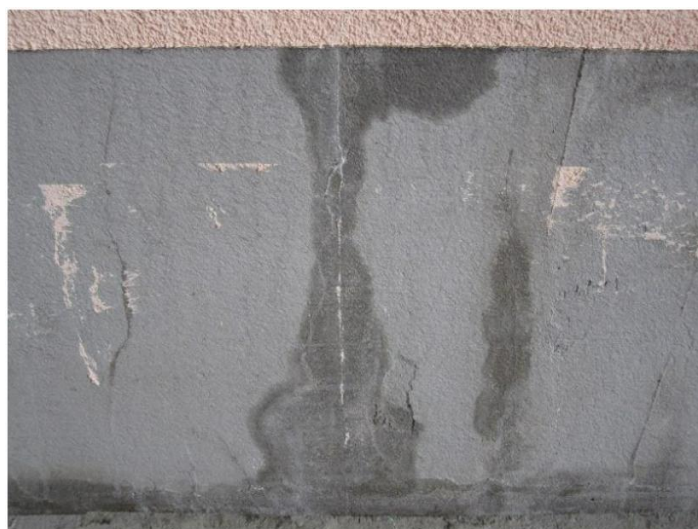
Figure 6: Detail of Various Defects on the Surface of the Base Coat Layer after the Test Cycles (Photo: ITC).
